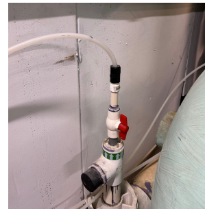
Tubing to be replaced
