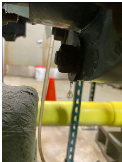
Previous sand filter flange leak
